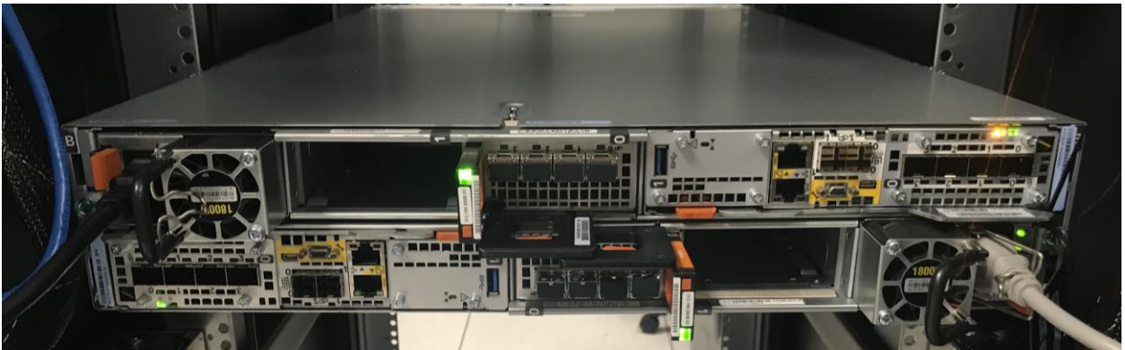
Figure 11. Rear of DPE (480/F, 680/F, 880/F)
